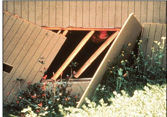
Example 2: Cripple wall failure where the floor shifted to the right..
