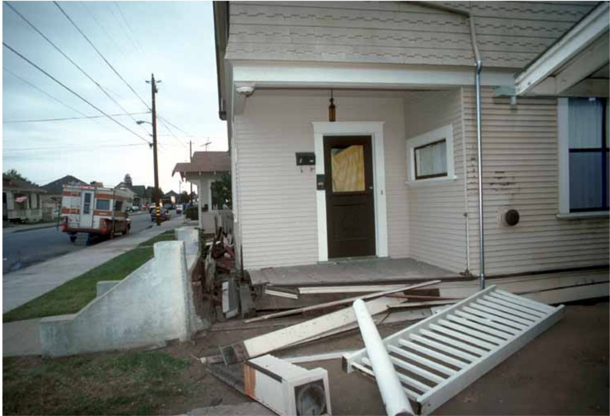
This house in Watsonville fell off its foundation because the cripple walls collapsed in the 1989 Loma Prieta earthquake. This would not have happened if the cripple walls had been retrofitted.
