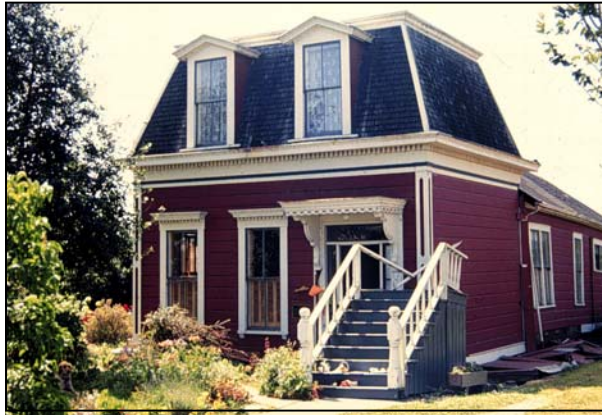
Example 1: Cripple wall failure; notice the location of the steps relative to the floor.
