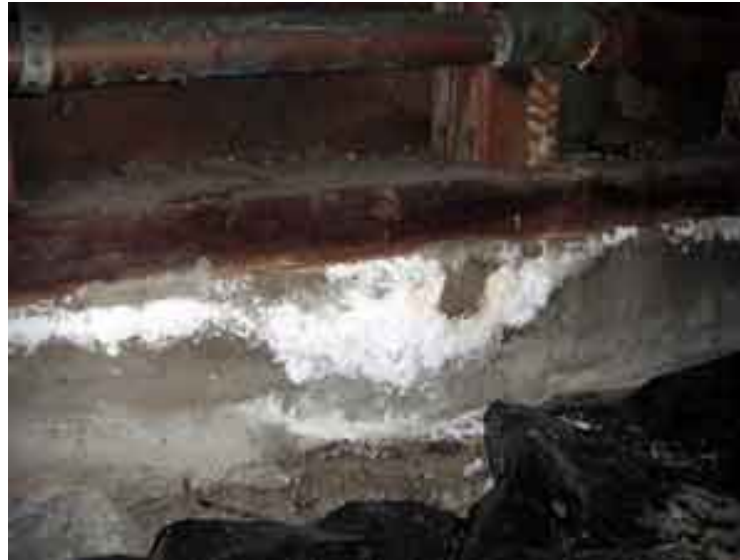
Figure 14 Typical Foundation with Efflorescence
