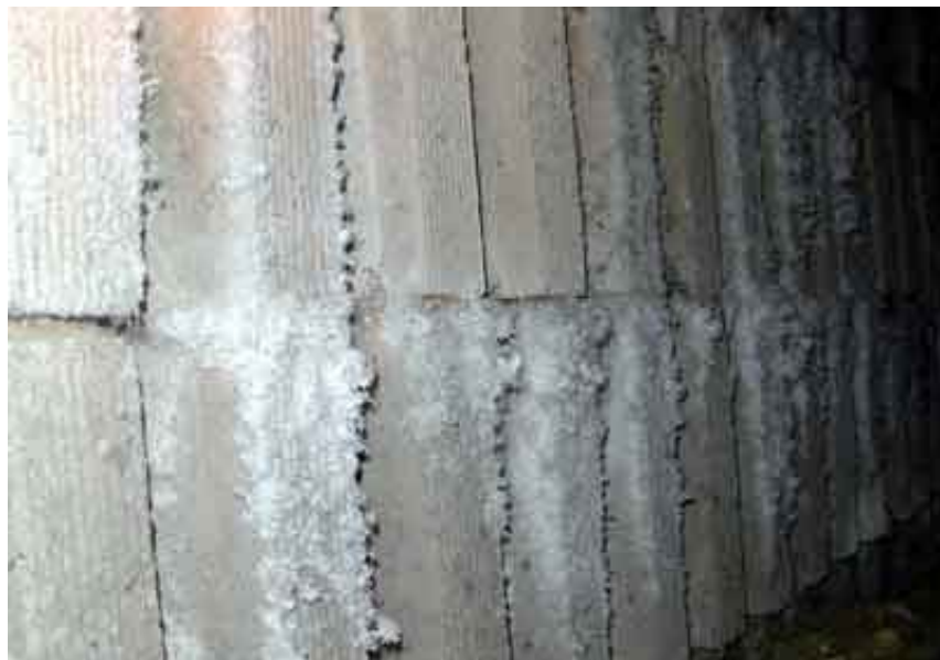
Figure 15 Masonry Blocks with Efflorescent Crystals
