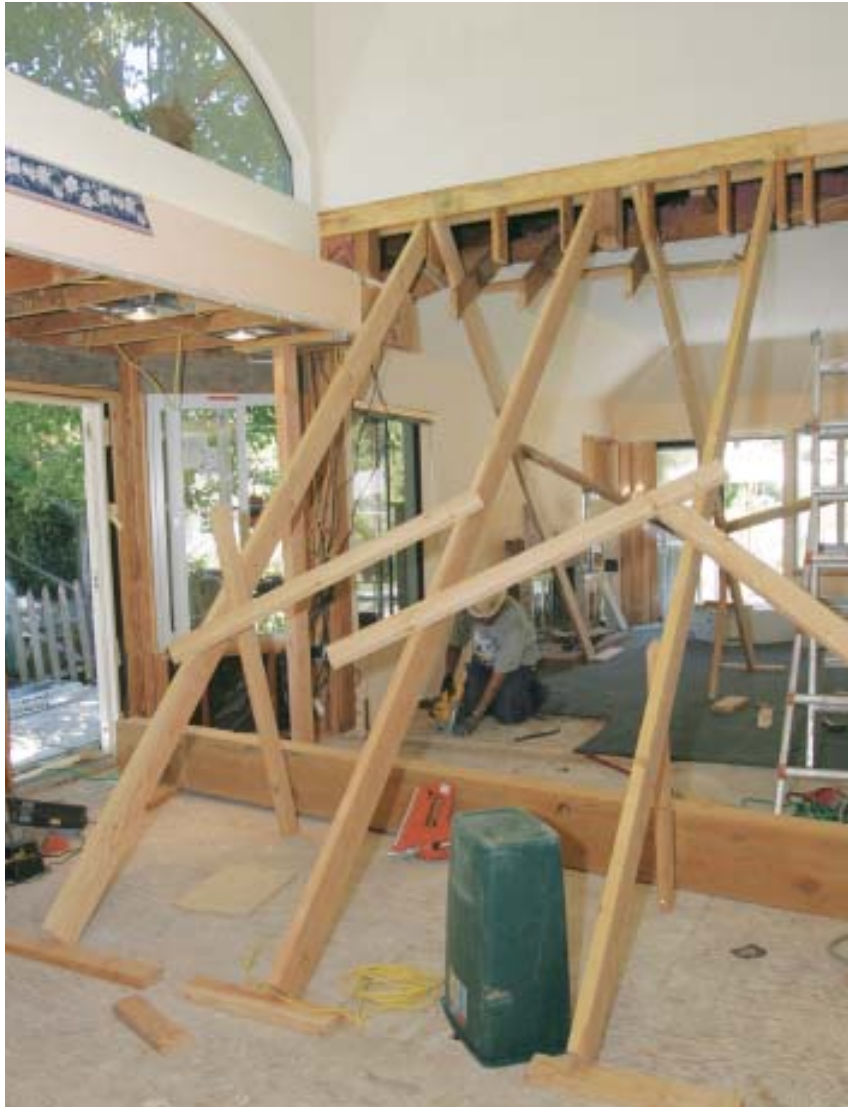
Figure 4. The author's crew used diagonal 2x6 braces to support the load above the shear wall while structural work was under way. To avoid having to maneuver the massive header through the braces, the workers prepositioned it on the floor and built the shoring around it.
