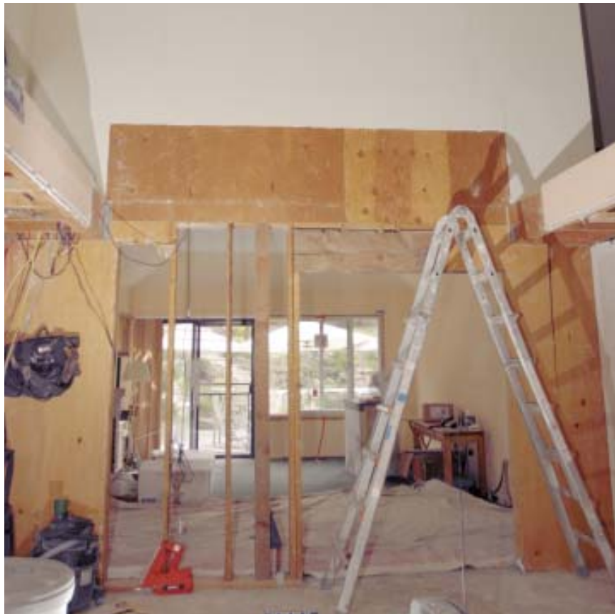
Figure 2. The wall between the two rooms was a shear wall; it's shown here after the soffit and some of the drywall and plywood shear sheathing were removed. The 4x6 post to the left of the opening is tied to the foundation by a heavy cast-in hold-down.
