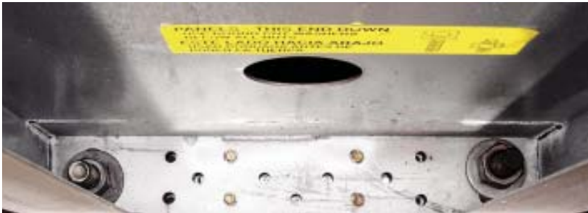
Figure 9. In this view down the open side of the shear panel, the installation is complete; nuts and washers are on the anchor rods, and screws pass through holes in the bearing plate into the joists and blocking below. The upper end of the panel (not visible) is screwed to the header above.
