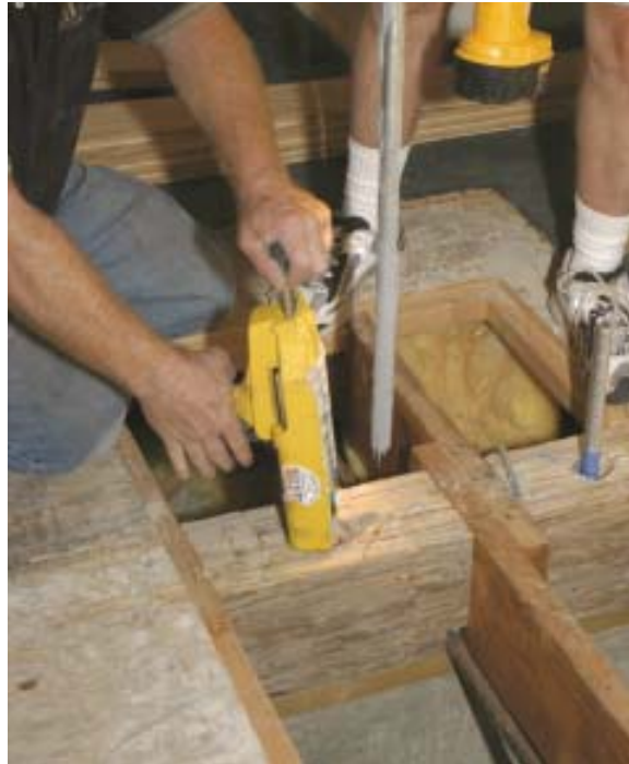
Figure 7. The rod on the right has already been installed through Parallam blocking and into an 18-inch-deep hole in the concrete foundation below. The glue-coated rod on the left was just removed from its hole so that the author could pump in an additional load of epoxy.
